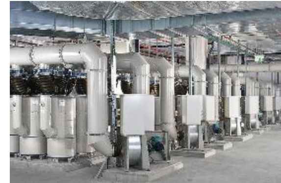
Filtration Batteries for Collective Shelters
